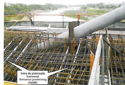
Figura 9. Vainas de pretensado transversal en la salida del tirante Figure 9. Transverse prestressing sheaths around the base of the stay
